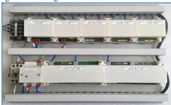
Figure 2. Integrated road street controller
