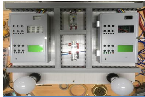
Figure7. Streetlight test bed
