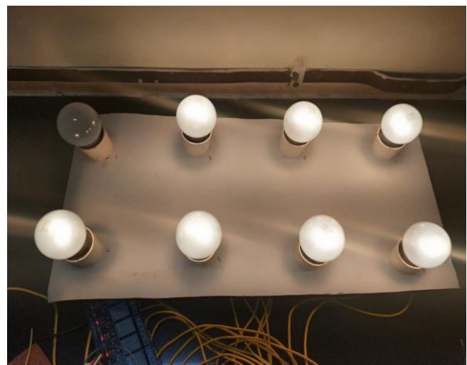
Fig. 12 Lamp 1 failed to glow for 1000 hours
